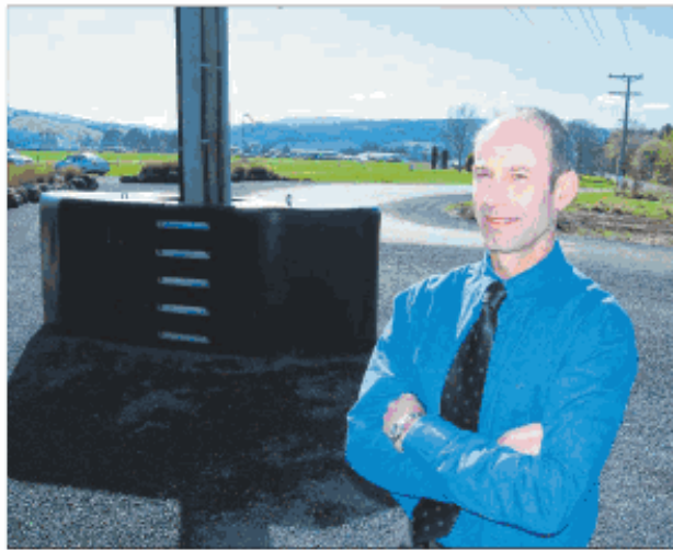
It's a wrap: Roothing engineer Evan Matheson says the South Island-first Raptor safety device on this power pole at the corner of Stedman and Wingatui Rds is a potentially good solution to an immovable problem.
